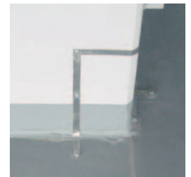
Ground connection of the conducting set
