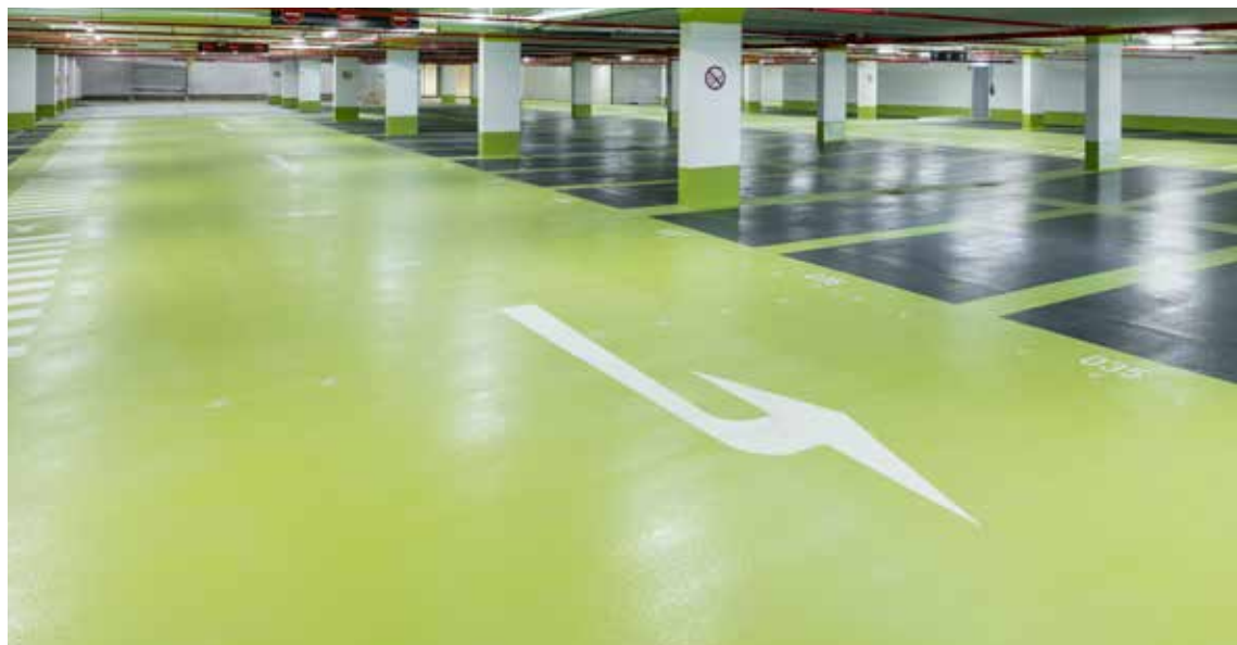
Cranachhöfe underground car park, Essen, DE Foto: Axel Hartmann
